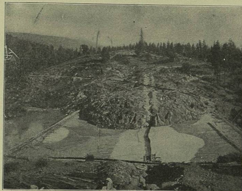
FIG. 79.—CRANE VALLEY DAM. SHOWING WOODEN FENCE, OR CENTER DIAPHRAGM, WHICH WAS CARRIED UP TO A HEIGHT OF 30 FEET ABOVE BED-ROCK.
