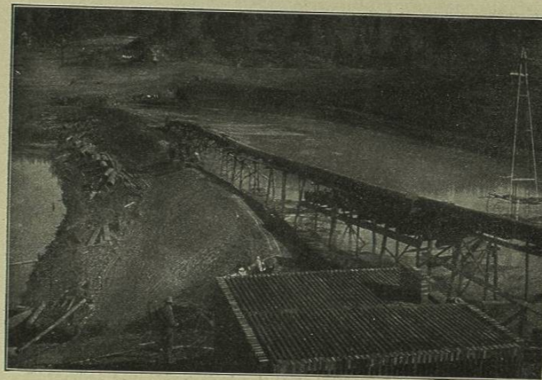
FIG. 86.—TOE LEVEL OF NORTH FACE, LAKE FRANCES DAM, AND INLET CRIB AT HEAD OF FIVE-FOOT OUTLET CULVERT.
