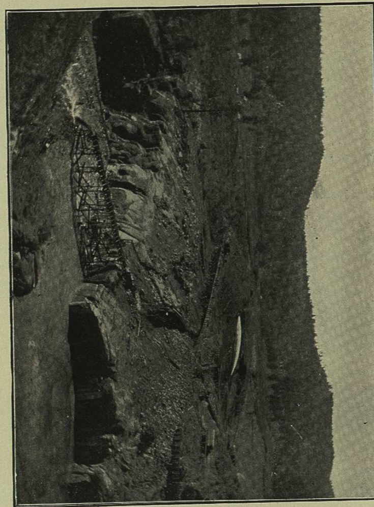
FIG. 107.—VIEW OF LOWER TOE FILLING, TERRACE DAM, COLORADO, SHOWING HYDRAULIC SLUICING IN BACKGROUND.
