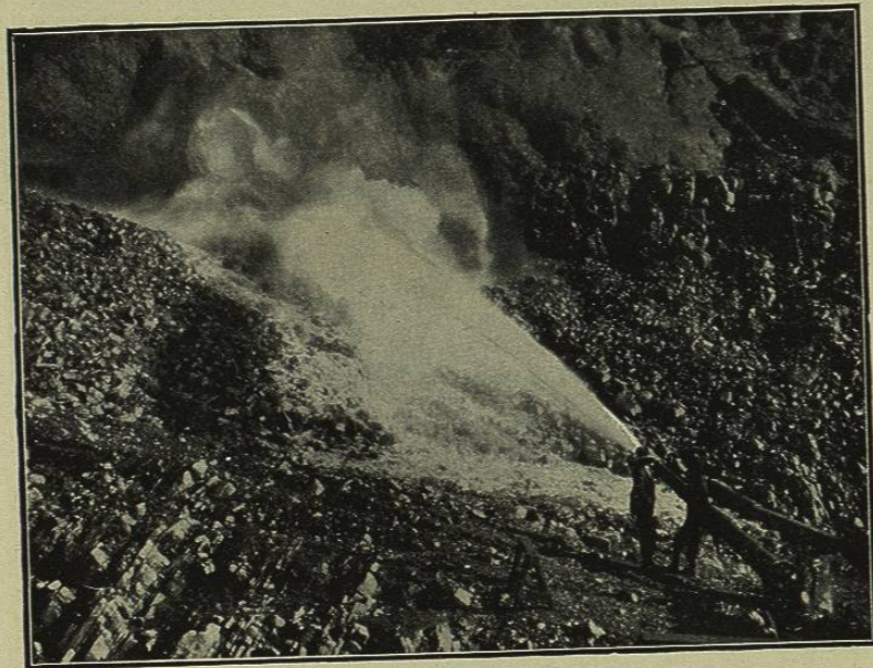
FIG. 117.—HYDRAULIC MONITOR WORKING ON LINE OF CONTACT BETWEEN LIMESTONE AND LAVA IN SPILLWAY CUT, NECAXA DAM, MEXICO.
