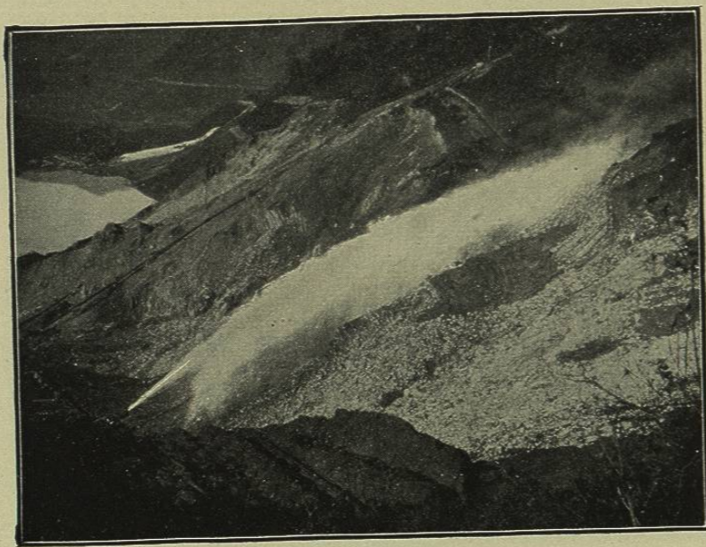
FIG. 115.—NECAXA DAM, MEXICO. HYDRAULIC MONITOR WORKING UNDER 180 POUNDS PRESSURE, 6-INCH NOZZLE, 30 SECOND-FEET OF WATER.
