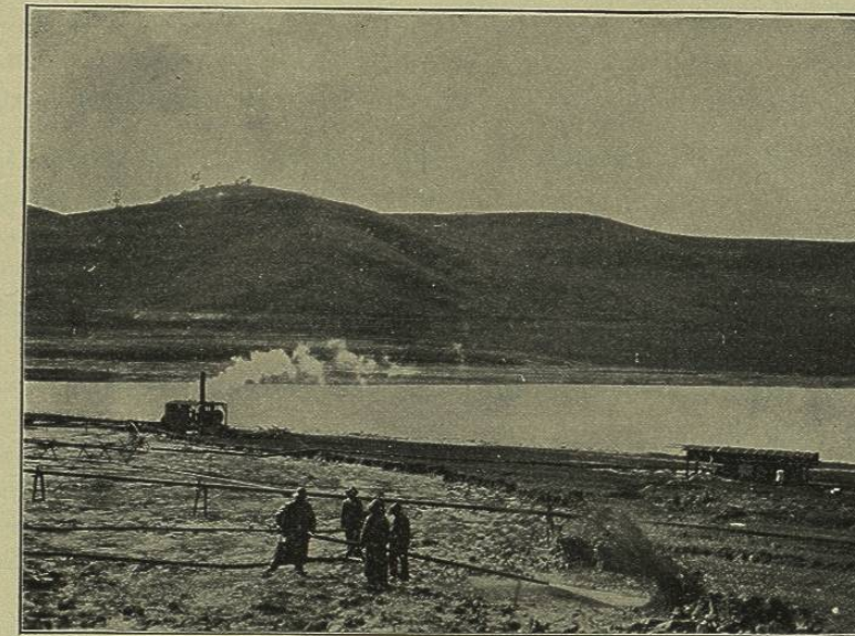
FIG. 136.—SILVER LAKE DAM, LOS ANGELES. THE EARTH, LOOSENED BY THE HYDRAULIC JET, IS CONVEYED TO THE PUMPING STATION SHOWN AND PUMPED TO THE DAM.
