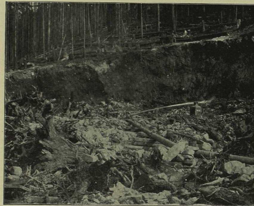
FIG. 145.—NORTHERN PACIFIC RAILWAY, HYDRAULIC-FILL CONSTRUCTION. VIEW IN PIT SHOWING HYDRAULIC GIANT IN ACTION.
