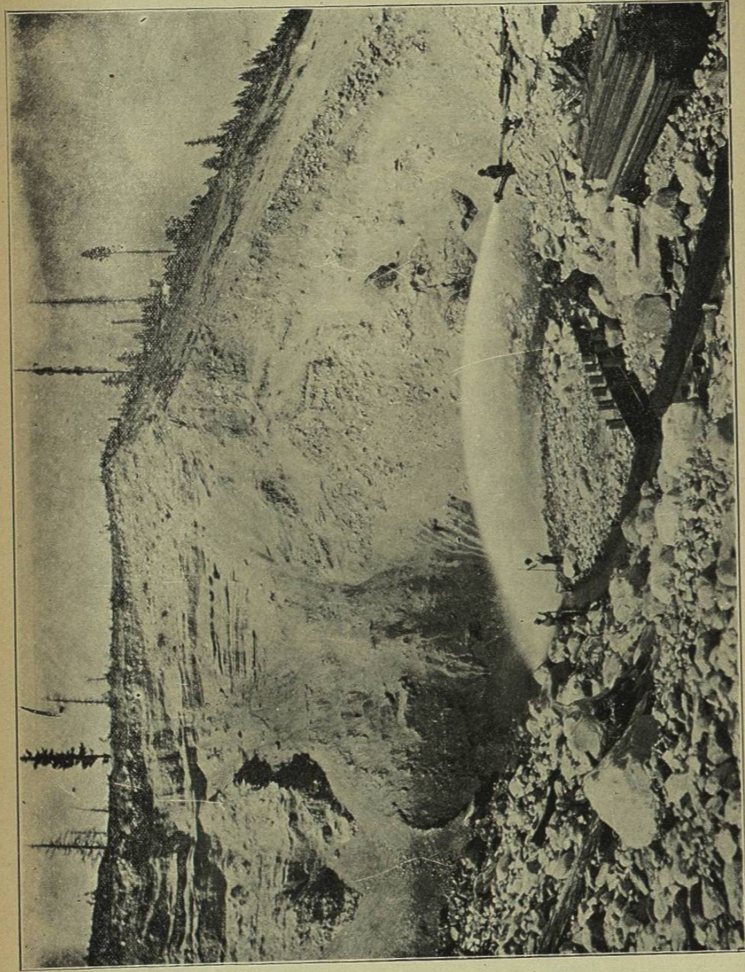
FIG. 140.—HYDRAULIC SLUICING, CANADIAN PACIFIC RAILWAY. VIEW OF PIT, AND HYDRAULIC GIANT AT WORK 194
