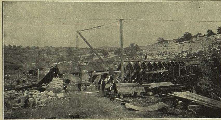
FIG. 294.—ASH FORK, ARIZONA, STEEL DAM, VIEW OF STEEL CONSTRUCTION FROM LOWER SIDE.
