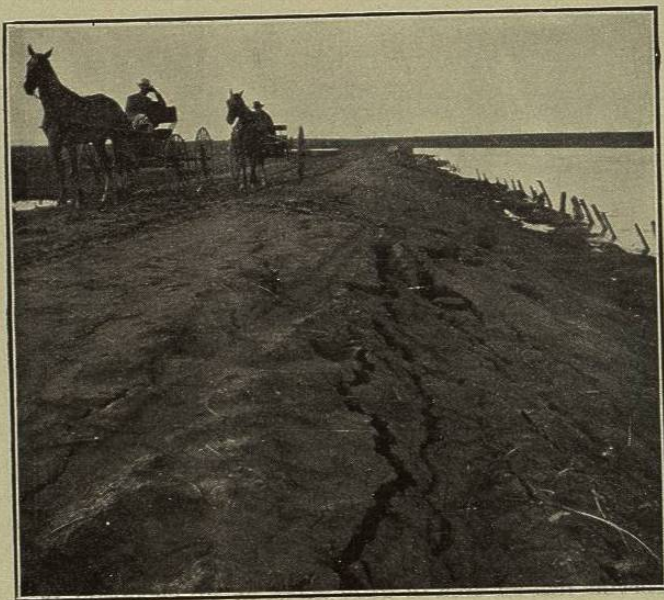
FIG. 333.—DOUGLAS LAKE DAM, COLORADO, SHOWING DANGEROUS SETTLEMENT CRACKS, DUE TO IMPROPER METHOD OF CONSTRUCTION.
